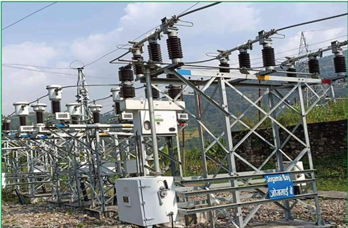
Jogmai/Jogmai cascade Bay at Godak substation
