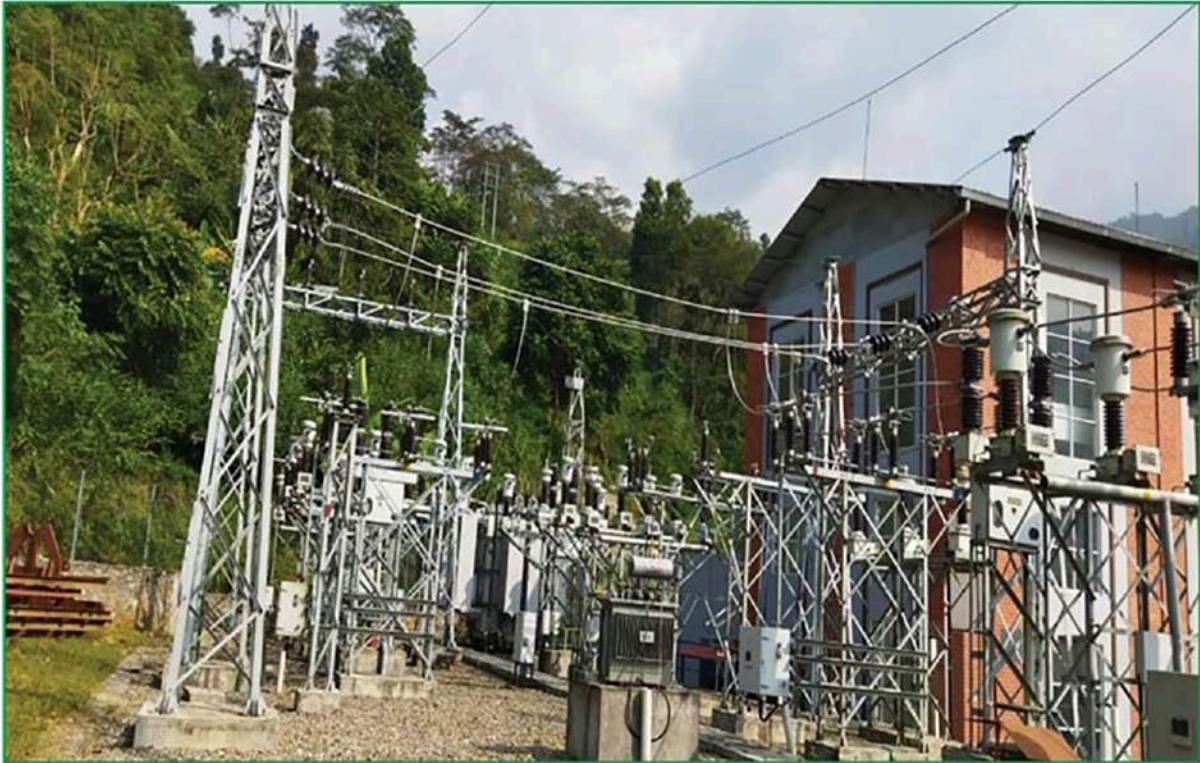
Loop in Loop out Provision of Cascade at Lower Jogmai Substation
